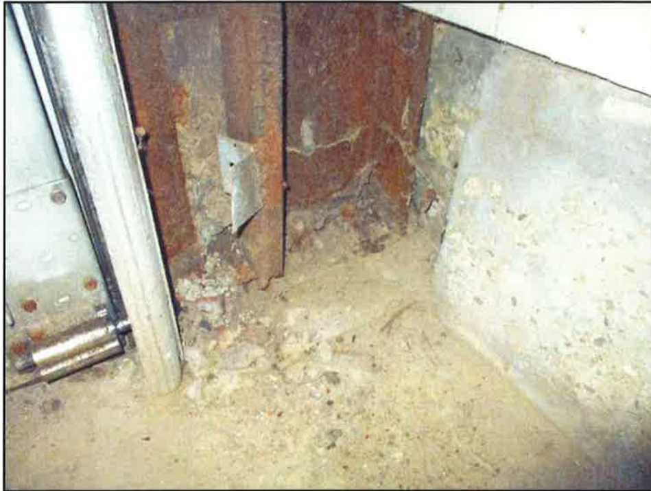
Photo 3: Localized severe section loss due to corrosion of bottom of exterior north wall framing end column.
