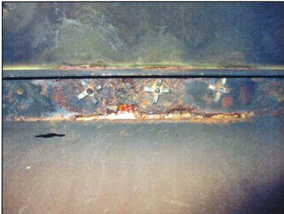
Photo 4: Localized section of severely corroded roof Z-purlin at interface of top flange and web View looking up.
