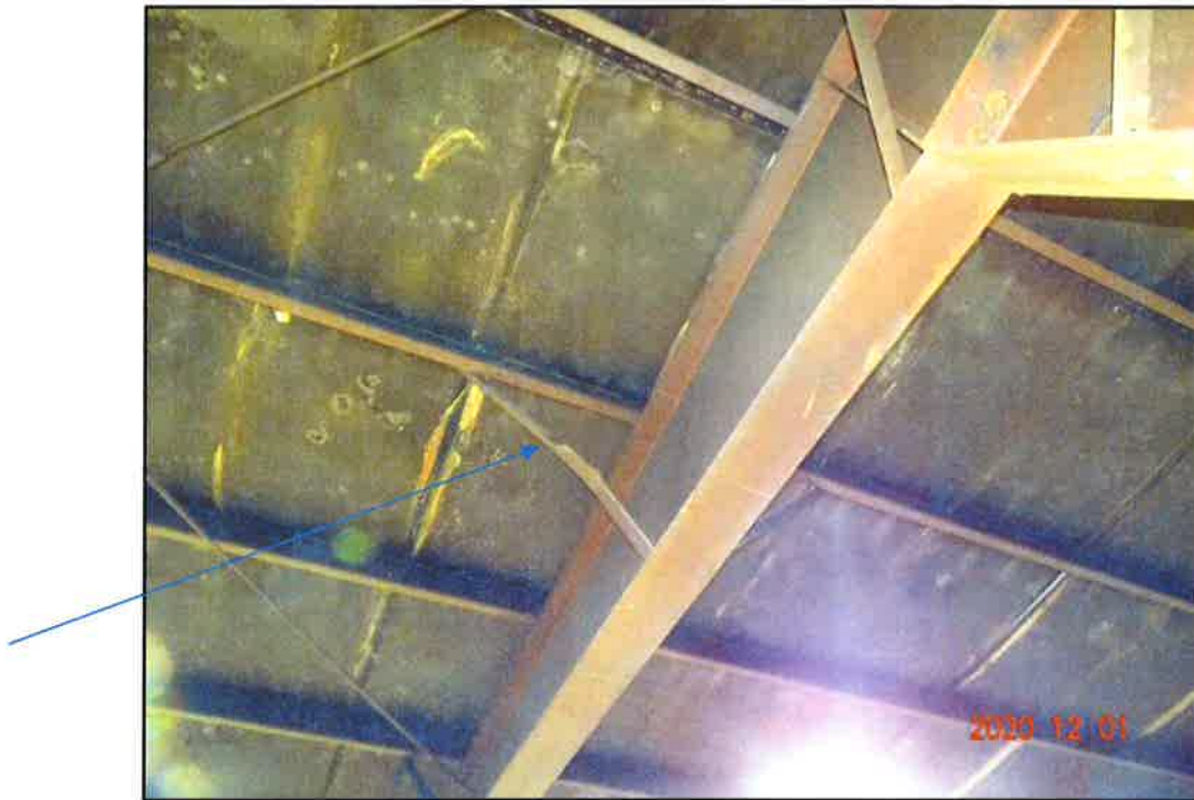
Photo 5: One of two diagonal roof strut with marked impact damage deformation.
