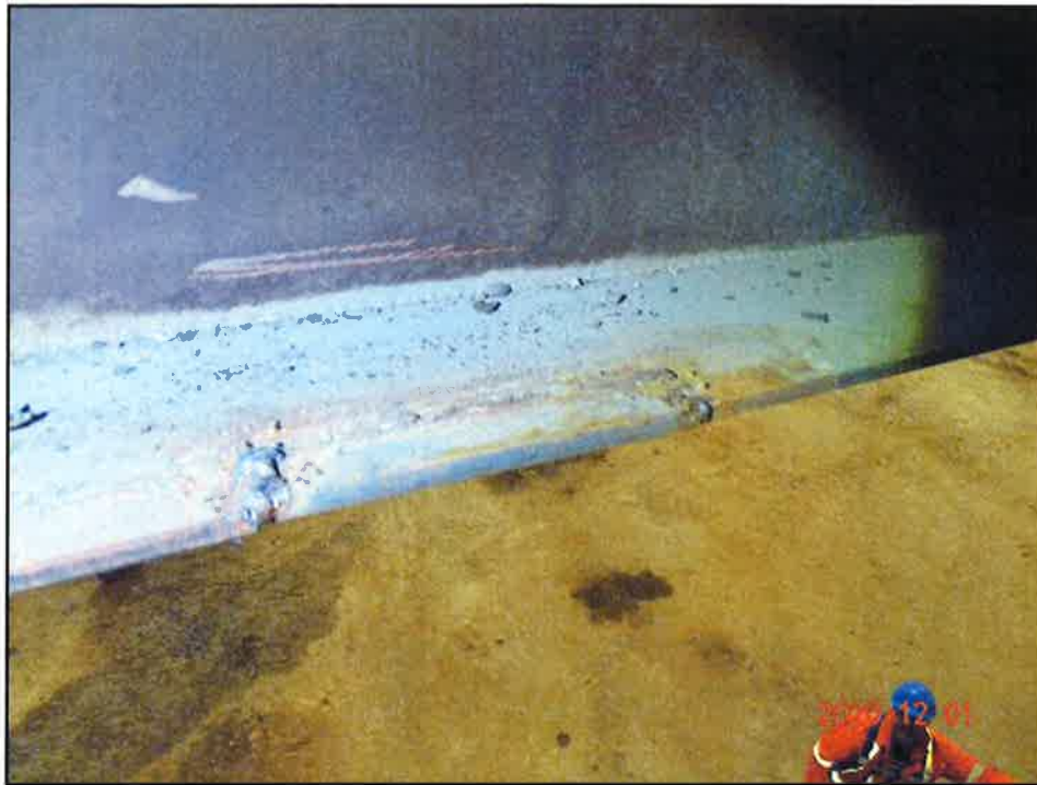
Photo 9: Coupon repair at rigid frame with incomplete joint penetration weld and requires coating with zinc rich primer.
