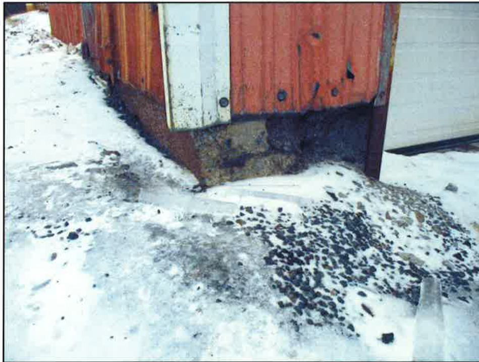
Photo 2: Isolated severe concrete foundation spalling at North-East building corner next to truck door.
