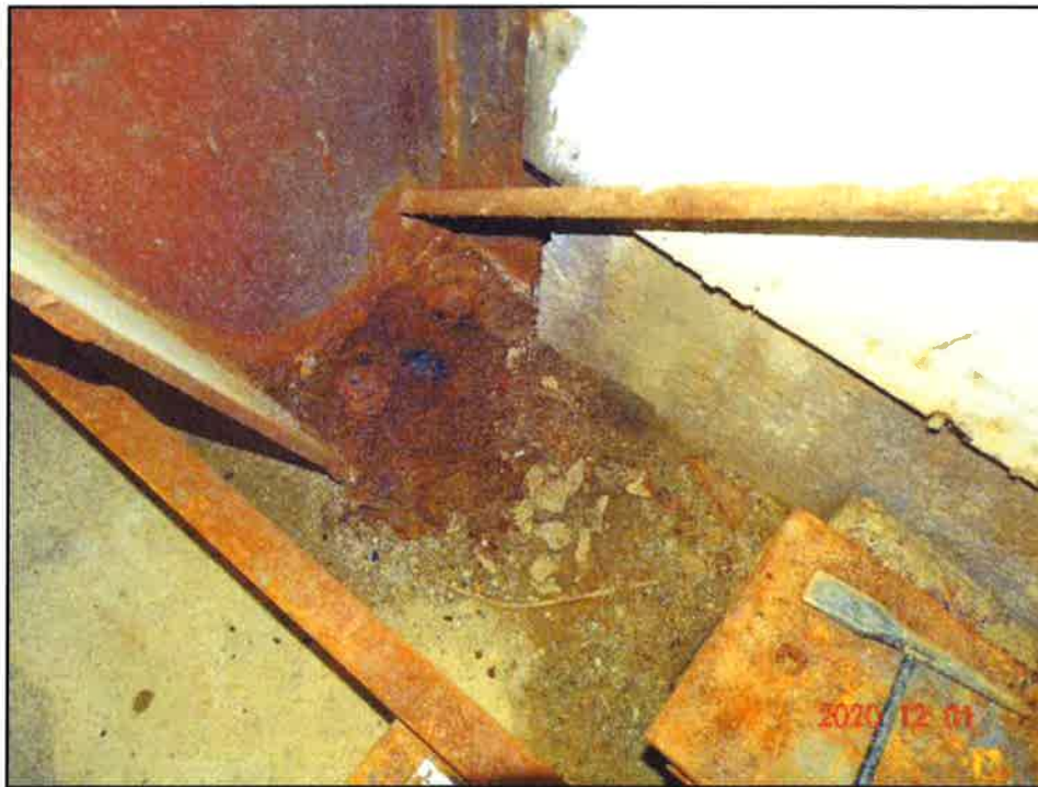
Photo 6: One of two Severely corroded rigid frame column base plate and anchor bolts along east wall
